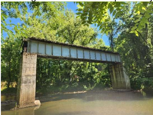
The remains of a bridge over the N. Fork Catawba River on a former spur off of CRR MP 207 (Sevier) into what was American Thread's Sevier plant.
