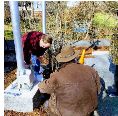
Jim Sutterlin and John Filippone putting the finishing touches on the base support.
