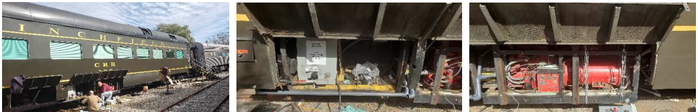
[Above left] Art Devoe and Gary Lombardi at work installing the gen set on Car 100. The other two photos are before and after shots of the compartment into which the motor fit.
